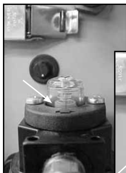
Figure 1: Button Down - Filter is Clean
